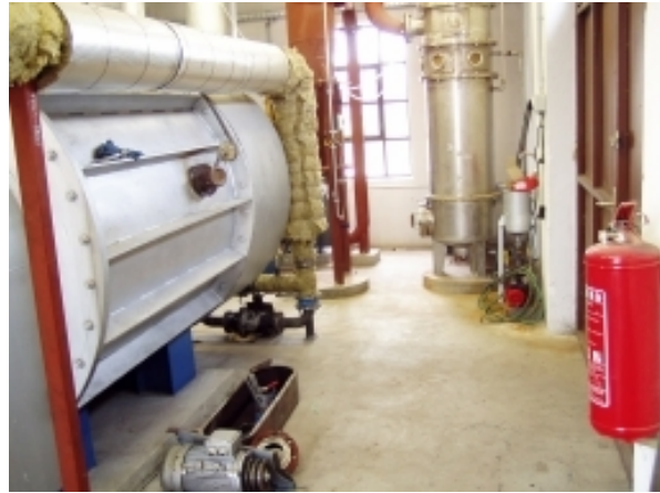
3R post burner and scrubber
