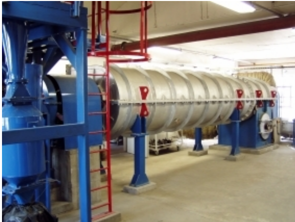
3R carbonization plant
